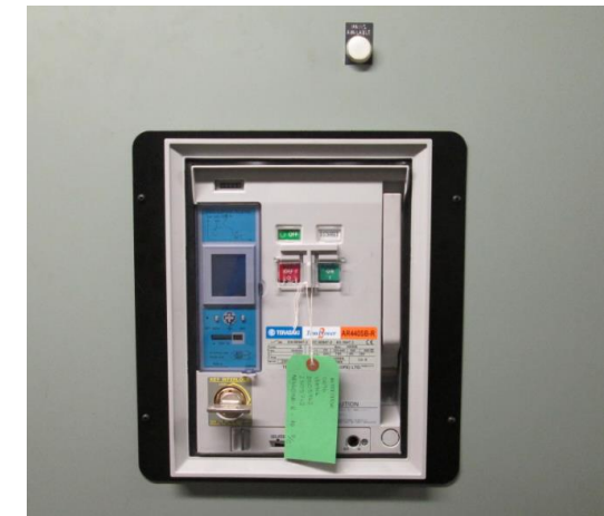
After: Retrofit ACB, protection relay with LCD
