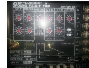
Before: Obsolete protection relay
