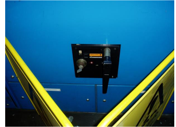
DA 4000 ACB: Access Restricted Due to Nuisance Tripping
