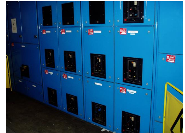
Obsolete Merlin Gerin Selpact ACBs
